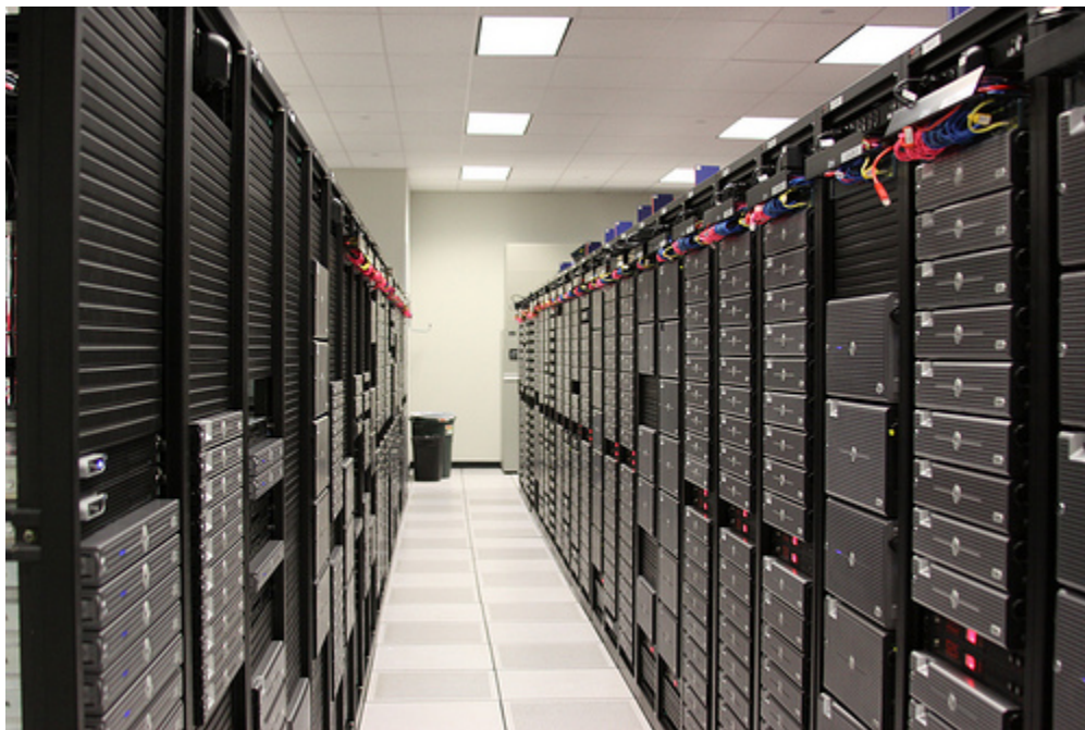
Servers inside a data center in Houston, Texas. [photo: The Planet]
